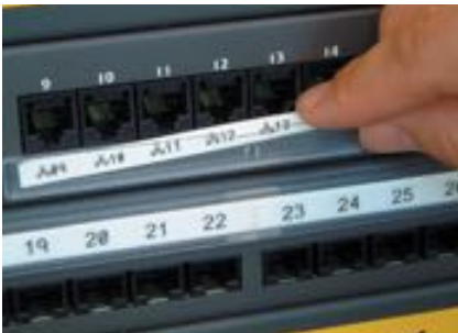
Punch Block & Patch Panel Labels
