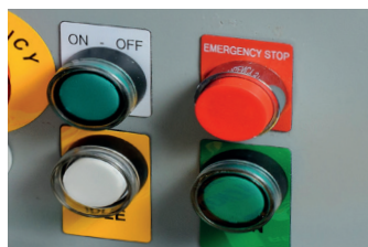
Control panel labels
