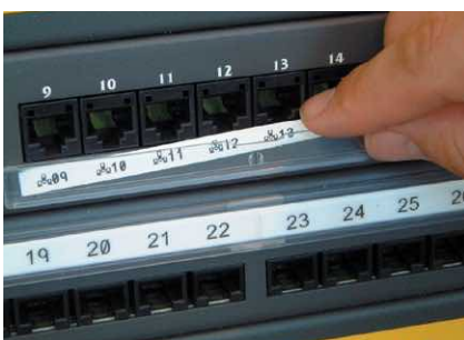
Punch block & patch panel labels
